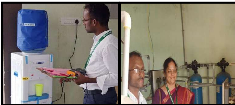
Water supply units and treatment facilities at SAWC, Vellore, Tamilnadu.
